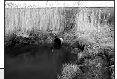
The undersized culvert (top) below the railroad track was replaced to increase tidal flow to the degraded upstream salt marsh.
