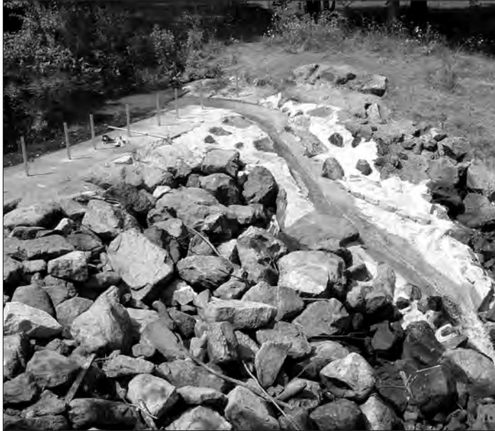
The recently installed chute on the spillway at Woolen Dam in Newbury enables fish migration.
