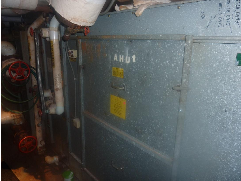
Photo 1 – Representative Air Handler
