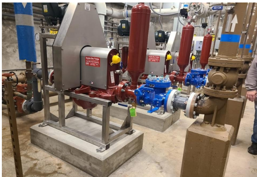
Figure 4: New Primary Sludge Double Disc Pumps and Variable Frequency Drives at the Edgartown WWTP
