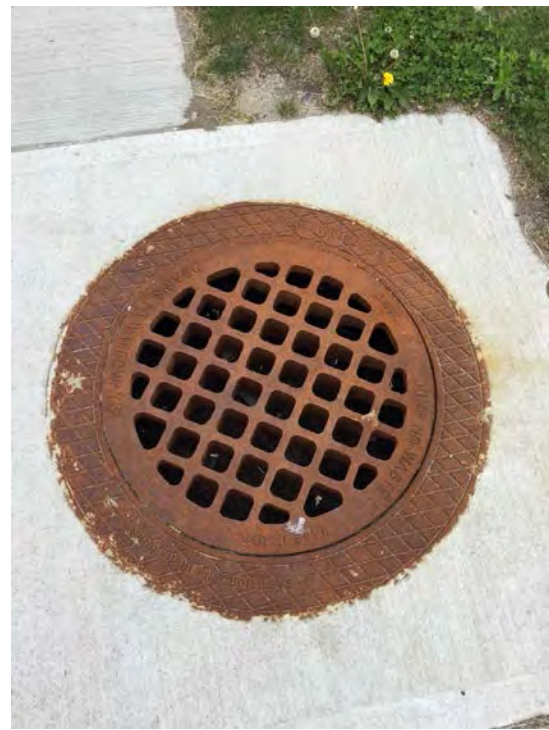
Site 11C, Morgan Street. Trees not installed.
