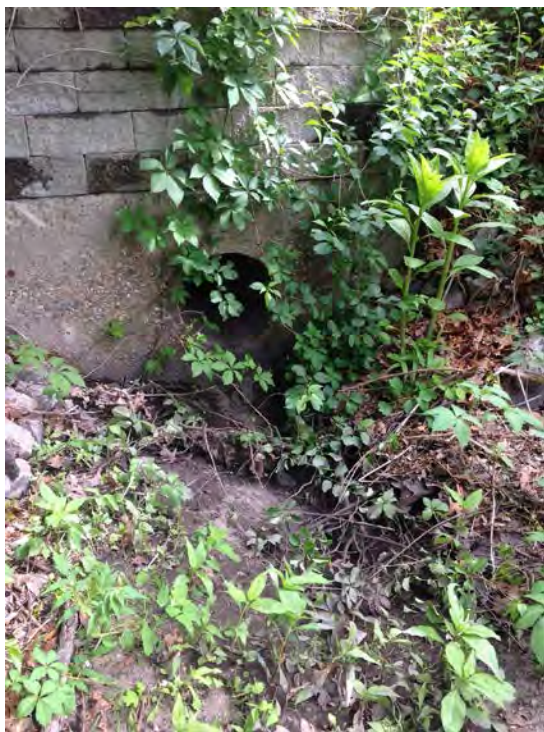
Forebay full of sediment.
