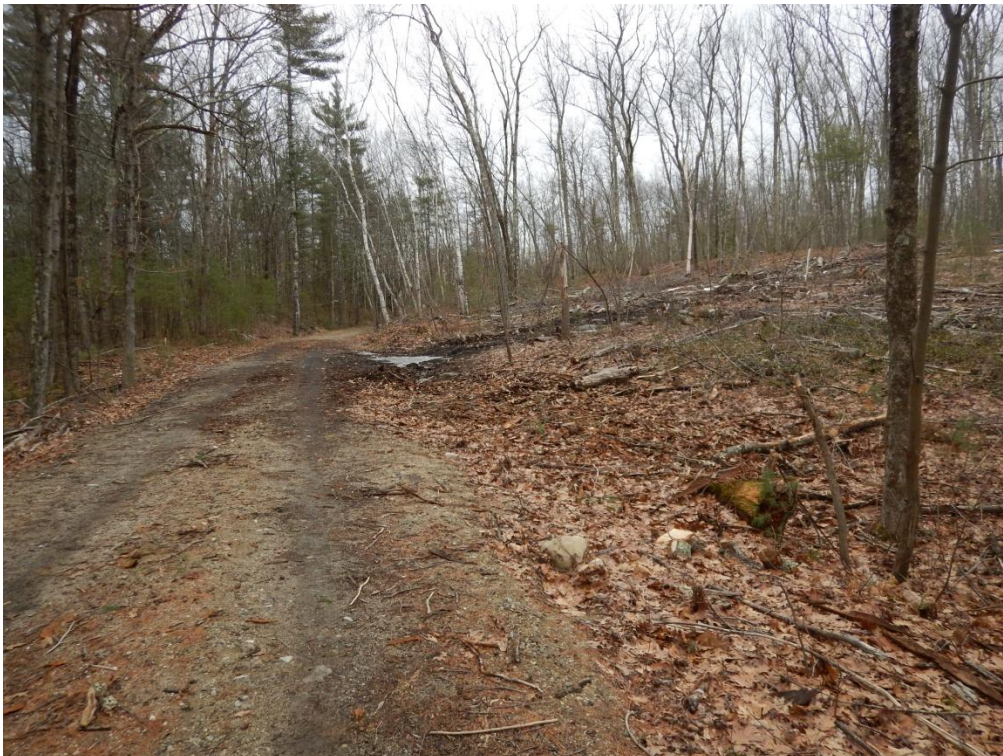
B. This was the primary landing for this operation. The restoration of this abandoned railroad bed by DCR heavy equipment crews recently now allows good access to this large chunk of DWSP property.
