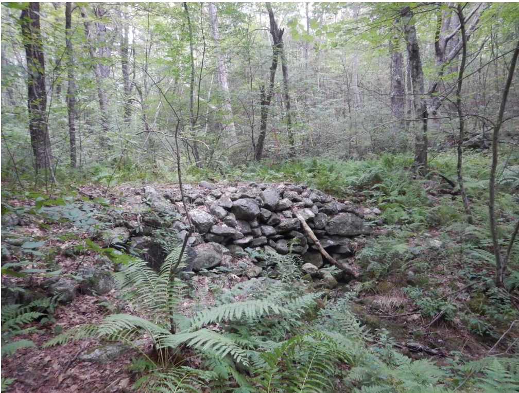
B. This is the stone bridge which will be used to cross the stream and access the sale area.
