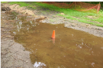
Image 1. Existing conditions after a rain event. Flooding and sediment build-up impact trail accessibility.
