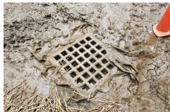
Image 2. Existing conditions after a rain event showing significant sediment build-up.
