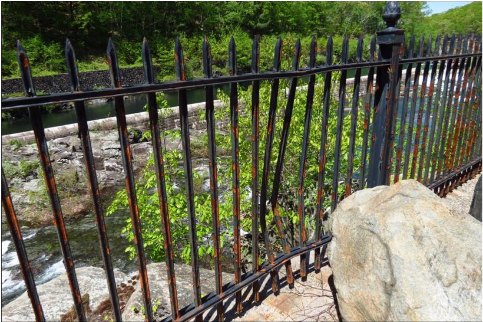
The fence has sustained damage in a number of places due to motor vehicle collisions.
