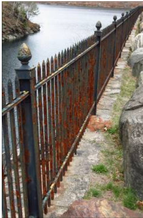
A section of fence showing the extensive rust and flaking of the protective paint covering.
