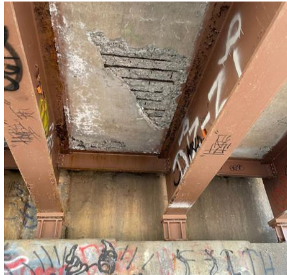
Widespread deck spalls with exposed reinforcing
