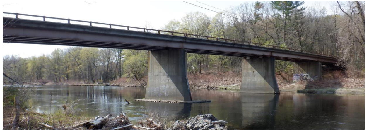
Existing piers have a history of scour/undermining
