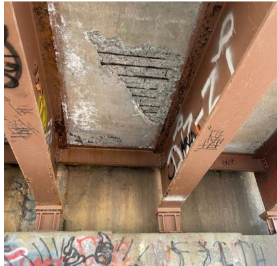
Widespread deck spalls with exposed reinforcing
