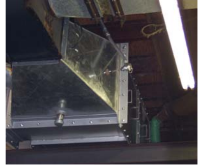
Delaware Valley's First Heat Exchanger
