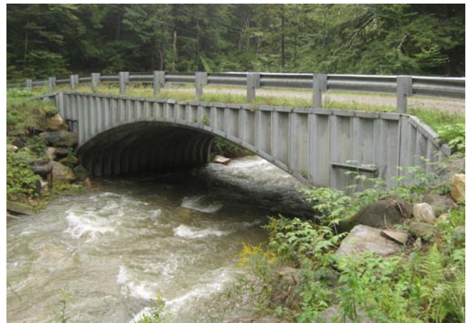
The upstream end of a bottomless culvert on Bronson Brook, that DER helped install, post-Tropical Storm Irene. Crossings of this type fared well in the high flows.
