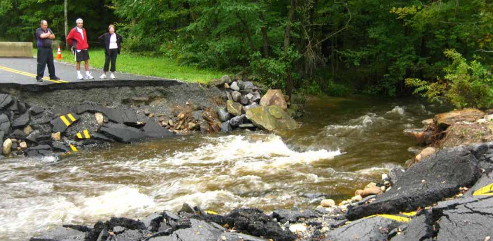
Undersized culvert on Benton Hill Road in Becket leads to a road being washed out during Hurricane Irene. Crossing was replaced in 2017 to meet the stream crossing standards with funds from a MEMA Hazard Mitigation Grant.
