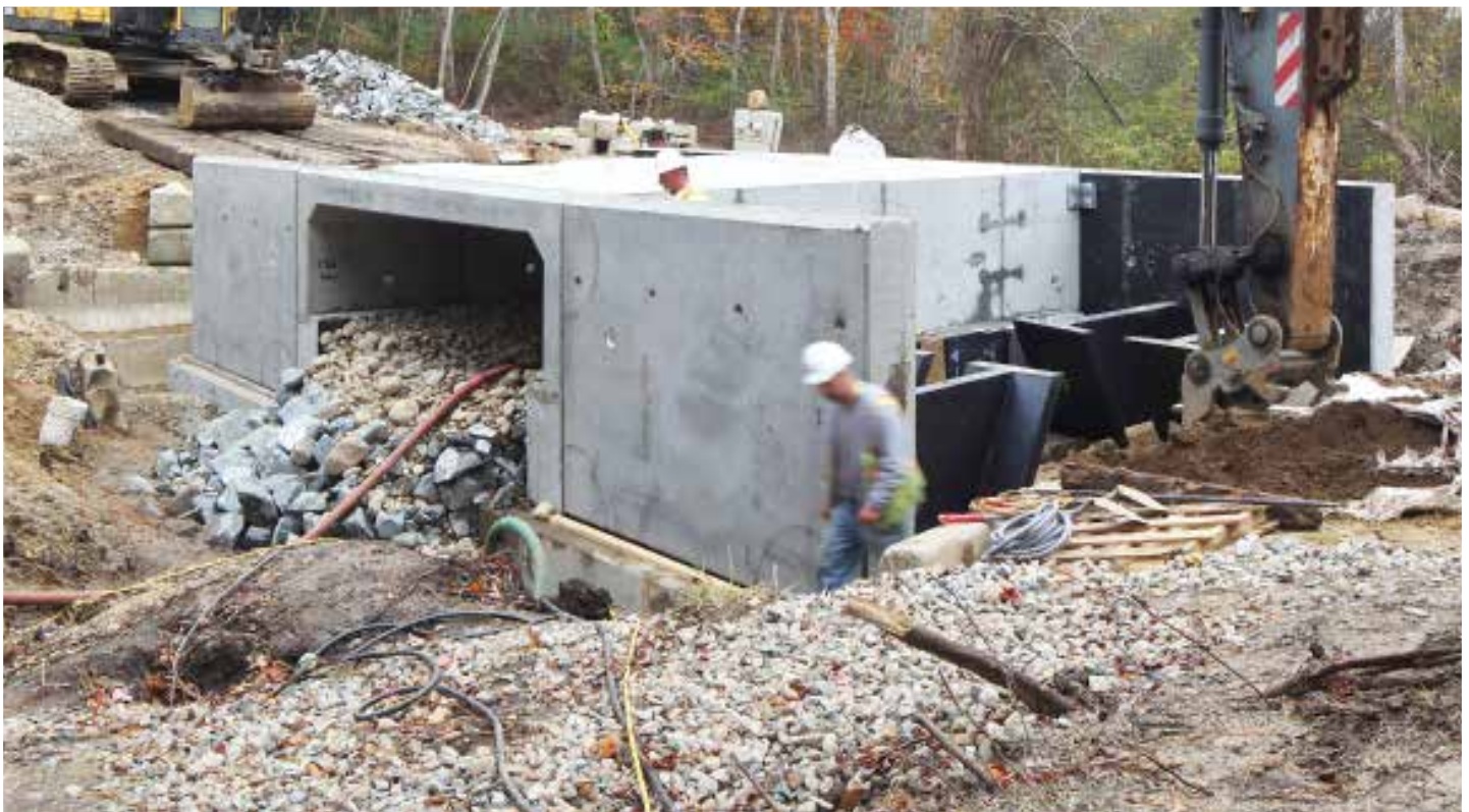
Replacement of the undersized culvert on Sampson's Mill Road in Mashpee is underway.
