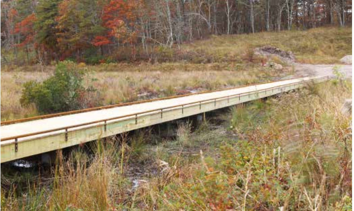
The Coonamessett River Restoration Project included construction of this new accessible boardwalk.
