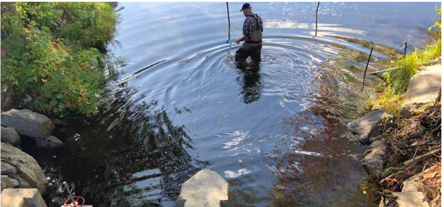
Installation of a stop log with a low flow outlet will enable low flow releases from Spectacle Pond.
