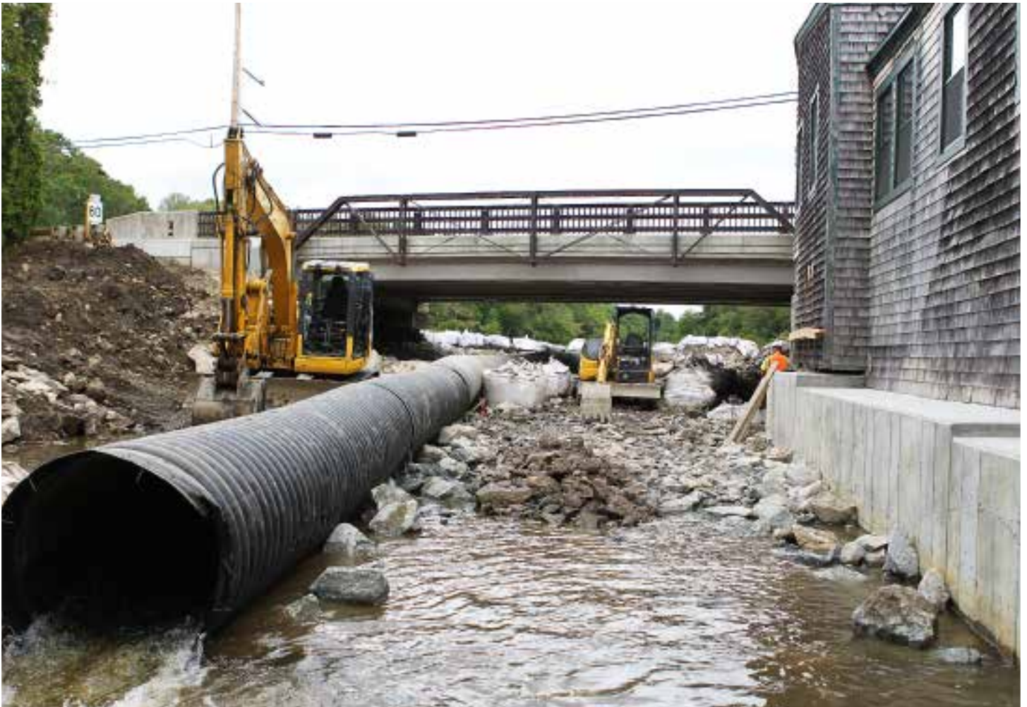
The removal of the Elm Street Dam reconnects 24 miles of river and restores habitat.
