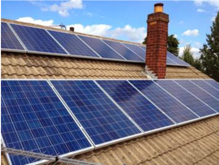
4 kW Class I Facility
