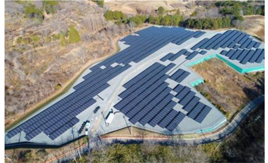
2 MW Class III Facility
