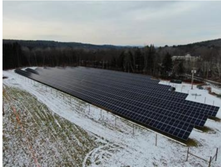
500 kW Class II Facility
