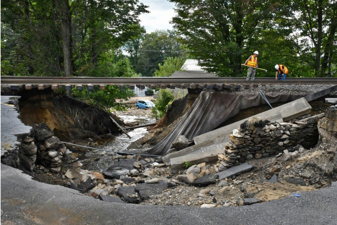
Workers measure MBTA tracks where heavy rains washed away the ground off Route 13 near Hamilton St. in Leominster. September 12, 2023 (Staff Photo Chris Christo/Boston Herald)
