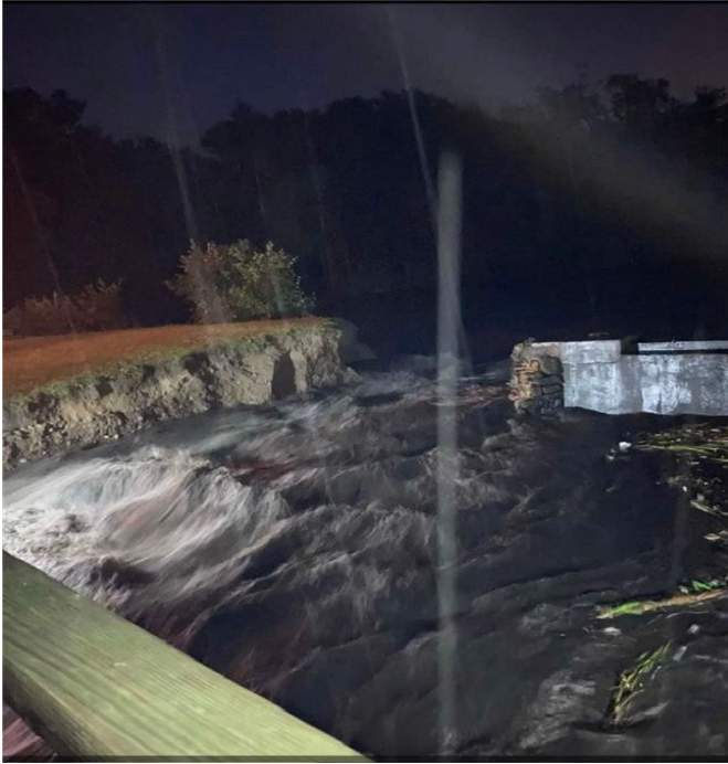
Barret Pond Dam overtopping and partial washout caused by flooding on September 11, 2023 (photo credit unknown)
