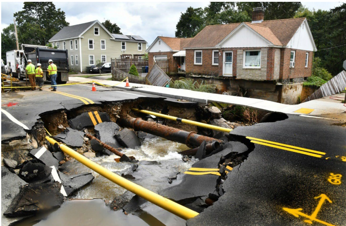
Flooding opened Pleasant St. and bared the foundation and made this home inhabitable at the intersection of Colburn St. in Leominster. September 12, 2023 (Photo credit, Chris Christo/Boston Herald)
