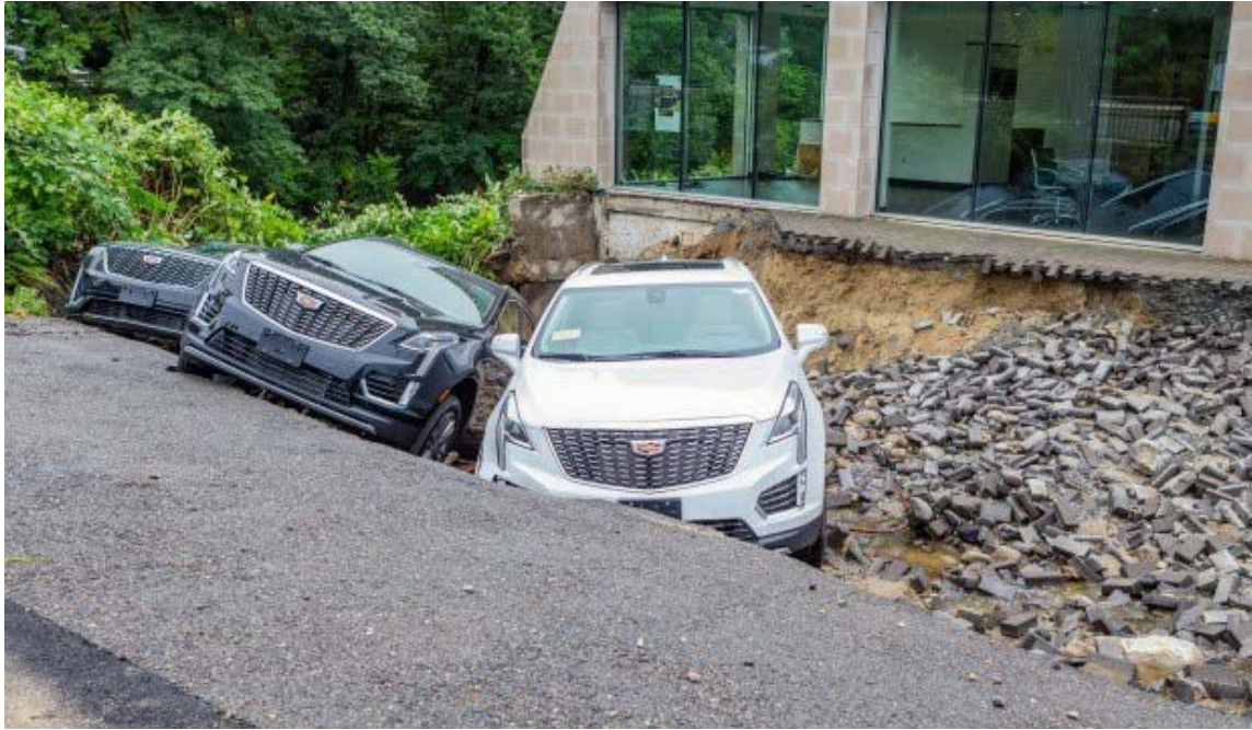
Large sinkhole at the Durand Cadillac dealership on Main St, in Leominster. (Photo credit GARY FOURNIER)
