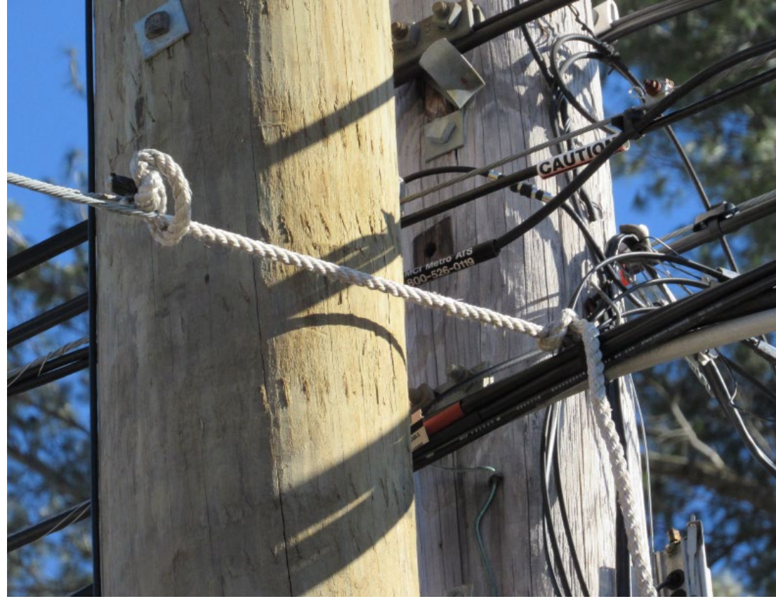
Double Pole Boxed – Two roadside communications and three field-side communications, creating complexity in the transfer process.
