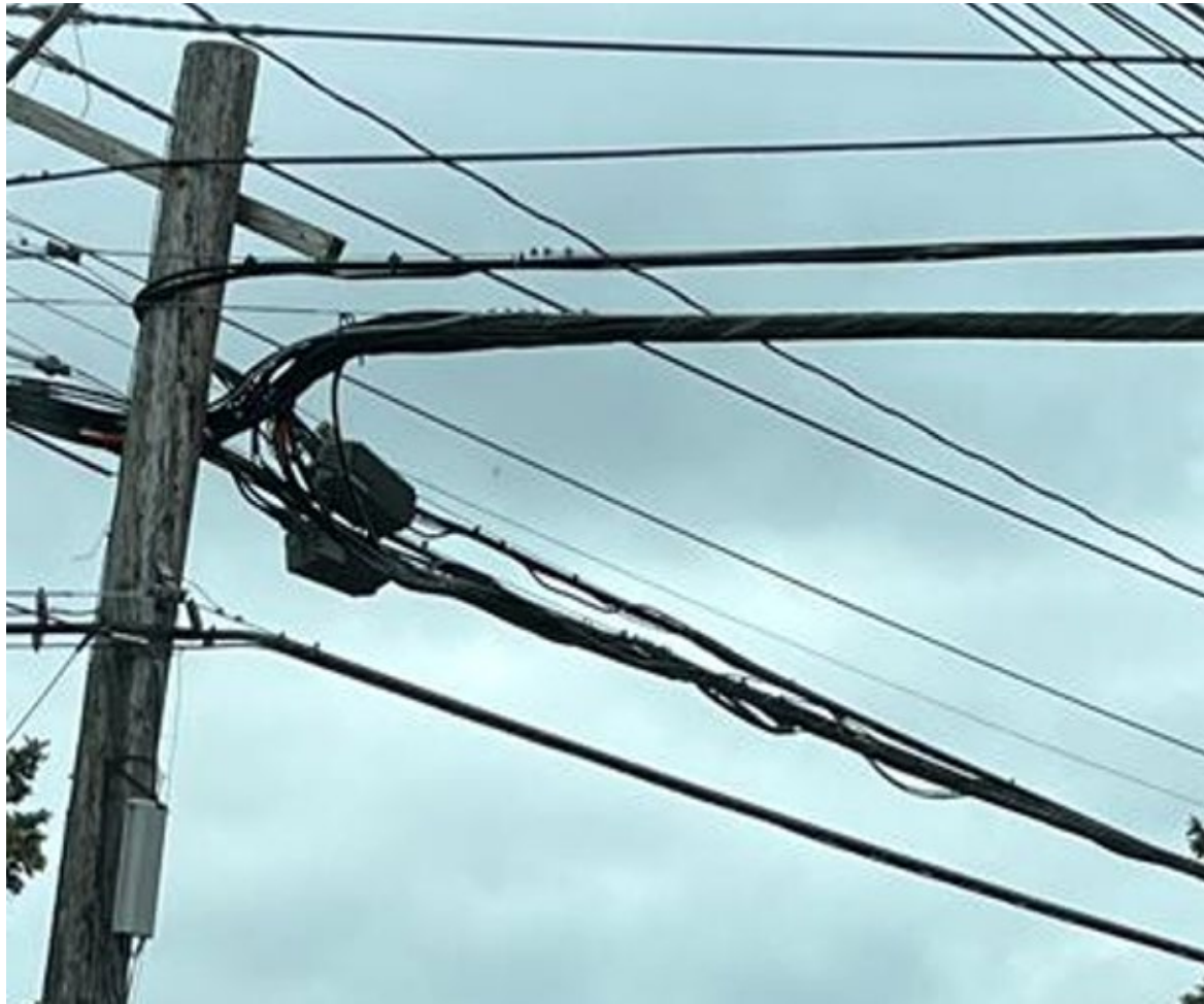
CATV over-lash at junction
