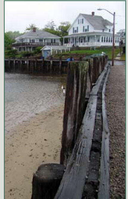
Seawall inside Wild Harbor at low tide on 1 June 2004. RPI photo.
