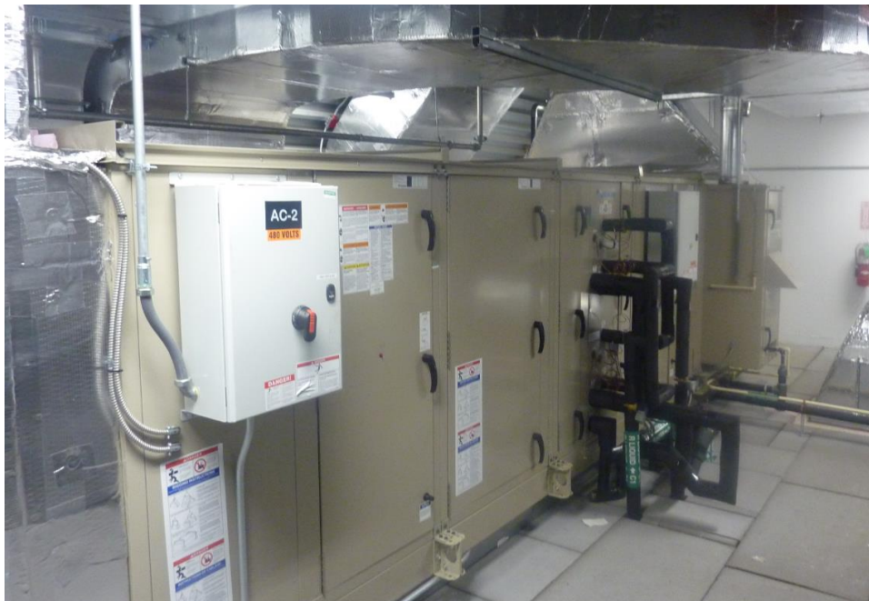
Photo 1 – Typical air handling unit
