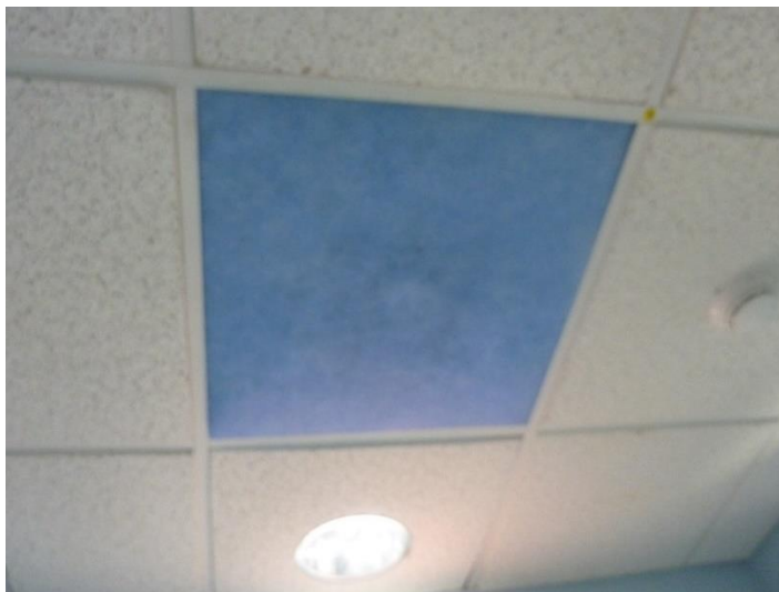
Photo 3 – Typical ceiling diffuser with filter fabric
