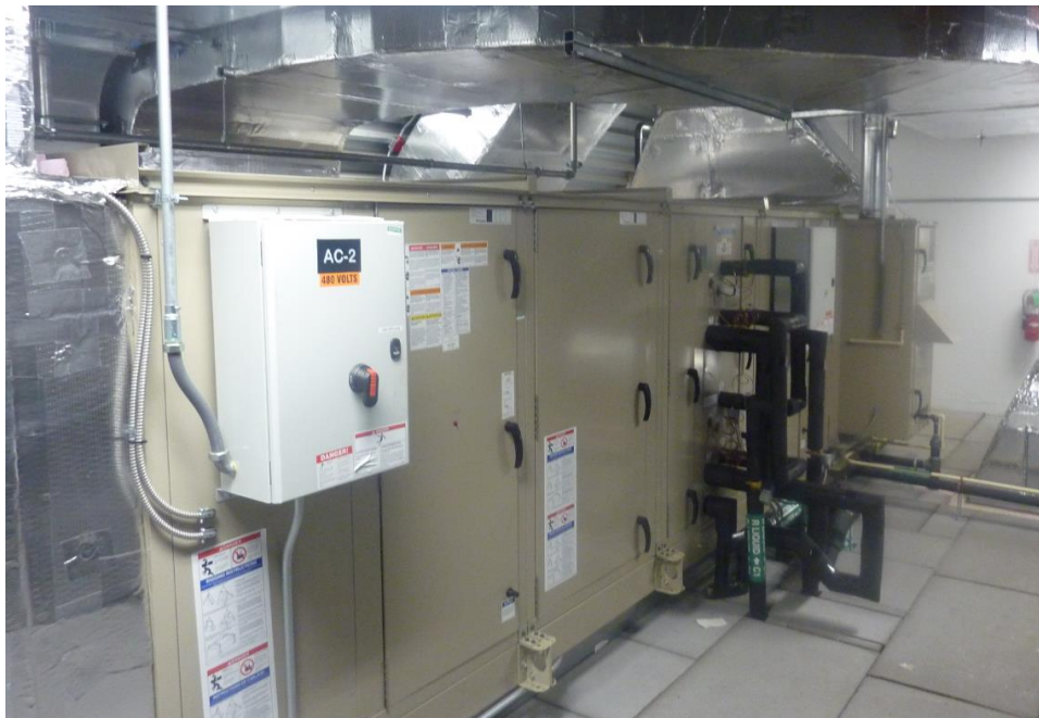
Photo 1 – Typical air handling unit
