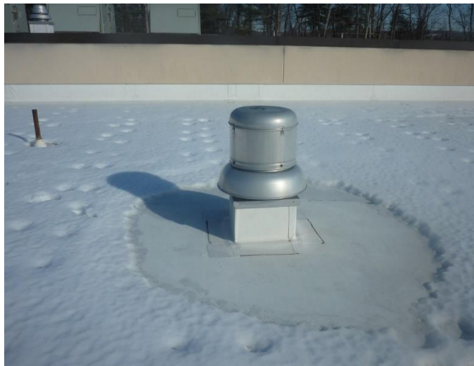
Photo 2 – Representative Exhaust Fans
