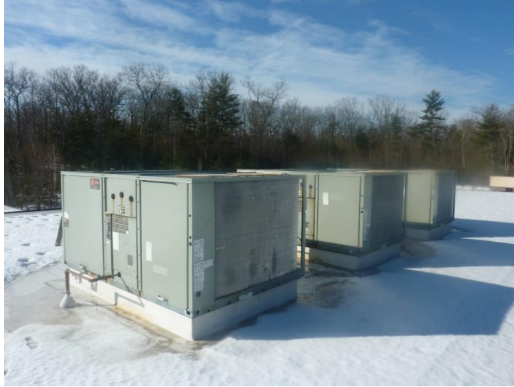
Photo 1 – Representative Rooftop Air Handlers
