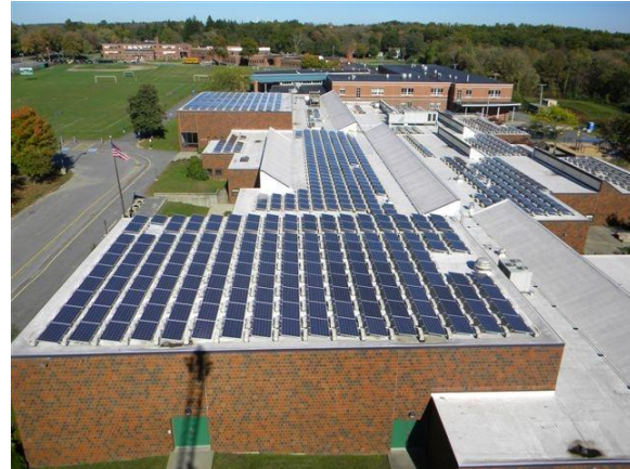
The Town of Sutton installed a 200 kW solar PV system, consisting of 898 Schott Solar PV panels, on the roof of the Simonian Early Learning Center.
