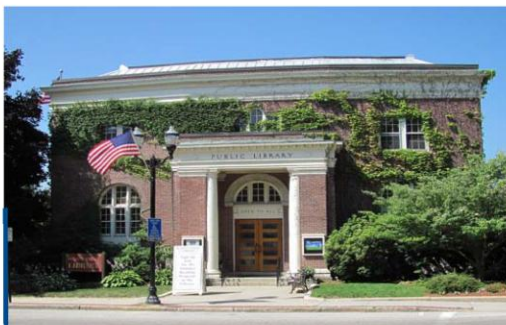
Left Photo: A worker installing new windows. Right Photo: Street view of the Hudson Public Library. *Photos courtesy of the Hudson Public Library
