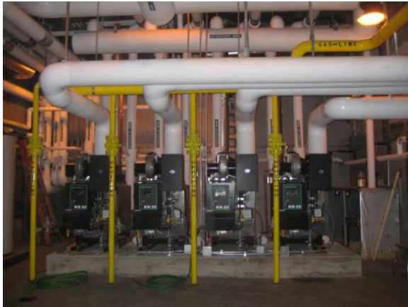
The Town of Saugus replaced the existing oil-fired boilers, hot water pumps and piping with four new gas high-efficiency condensing hot water boilers, three new hot water pumps and new piping at the Belmonte Middle School.
