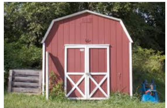
Figure 7: Outbuilding constructed in 1975 is located 55 feet west of the back of the house. This structure will be removed as part of the demolition project.
