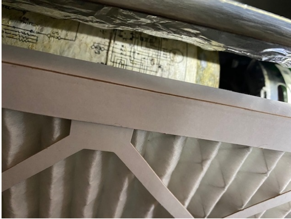
Photograph 3 Gap between Filter Frame and FCU Filter Rack in Room 422, 50 State Street, Springfield, Massachusetts.
