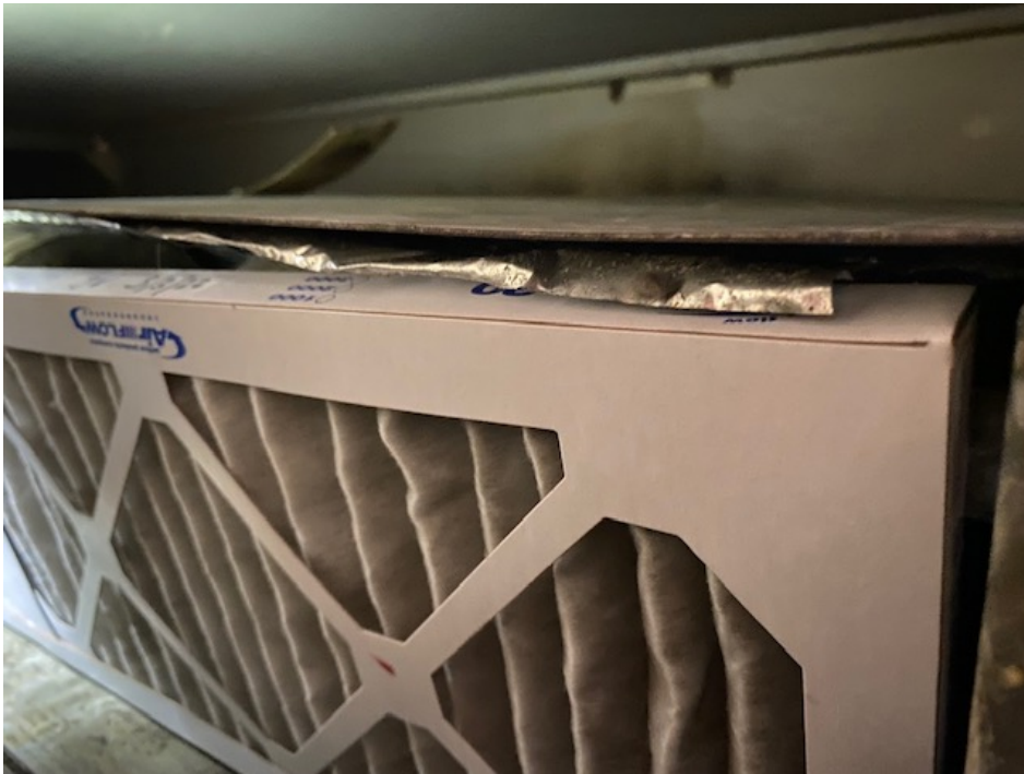
Photograph 4 Gap between Filter Frame and FCU Filter Rack in Jury Pool 446, 50 State Street, Springfield, Massachusetts.
