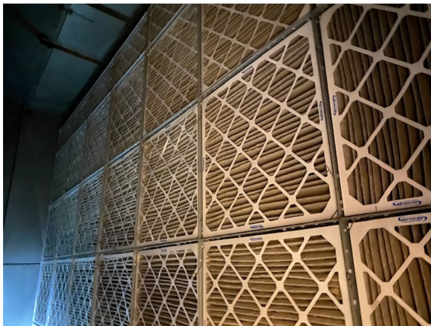
Photograph 1 MERV-13 Filters AC-1, 50 State Street, Springfield, Massachusetts.
