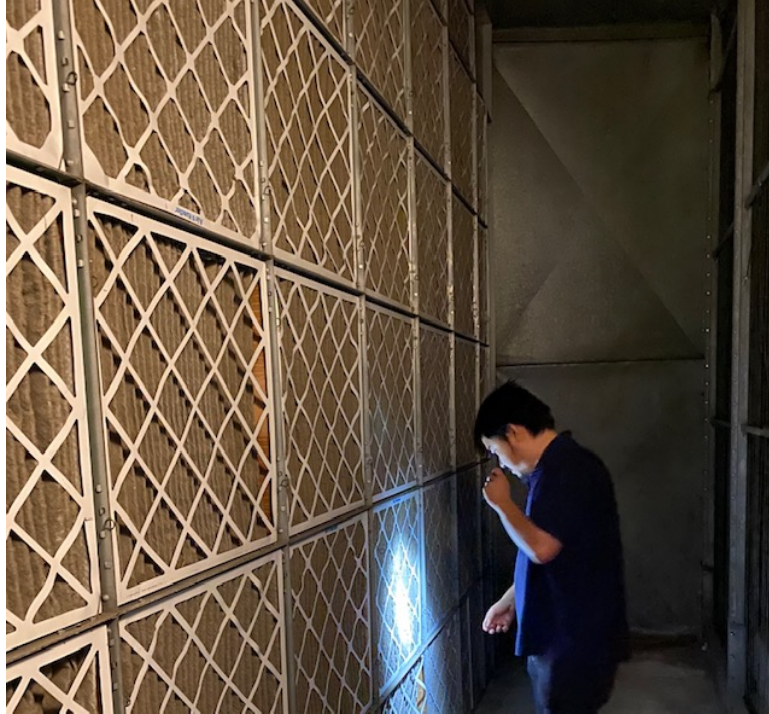
Photograph 2 MERV-13 Filters AC-4, 50 State Street, Springfield, Massachusetts.
