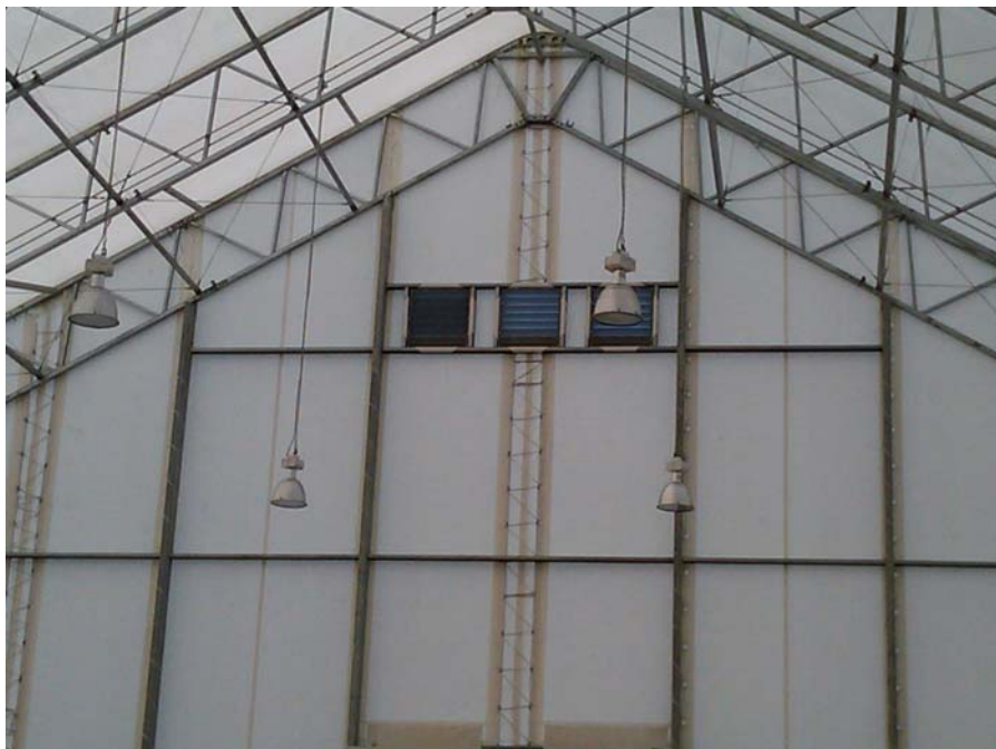
Passive louvered vents In The Expo Center
