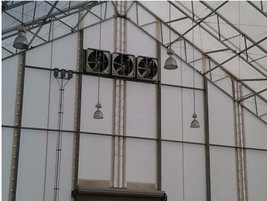
Exhaust fans in the Expo Center
