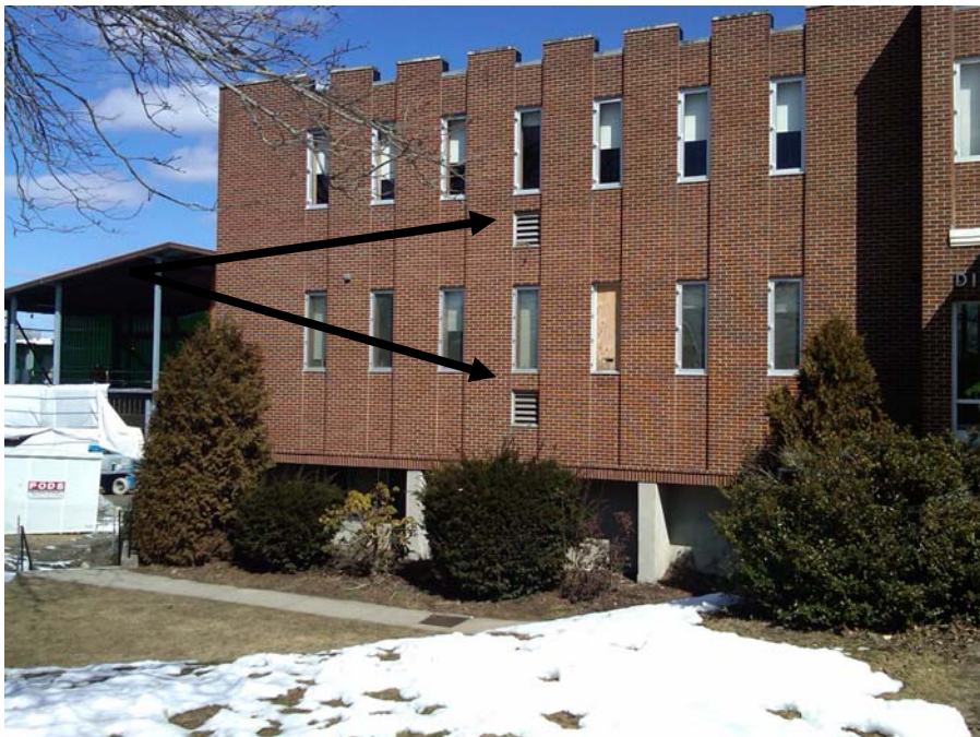
Example of univent fresh air intakes (arrows)
