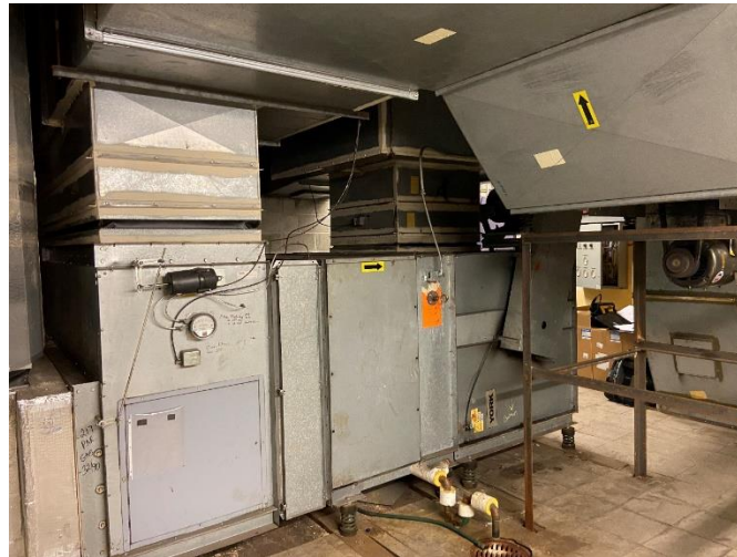
Photo 1 – Representative Air Handler
