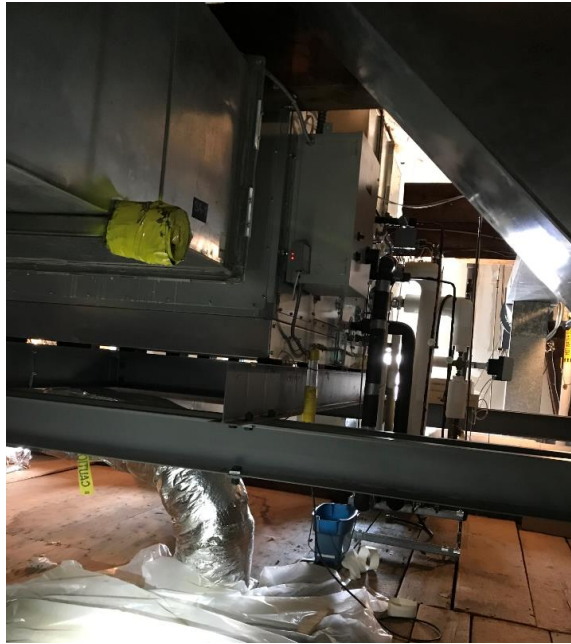
Photo 1 – Air Handler AC-1
