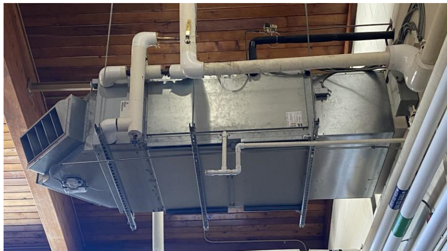
Photo 1 – Representative Air Handler
