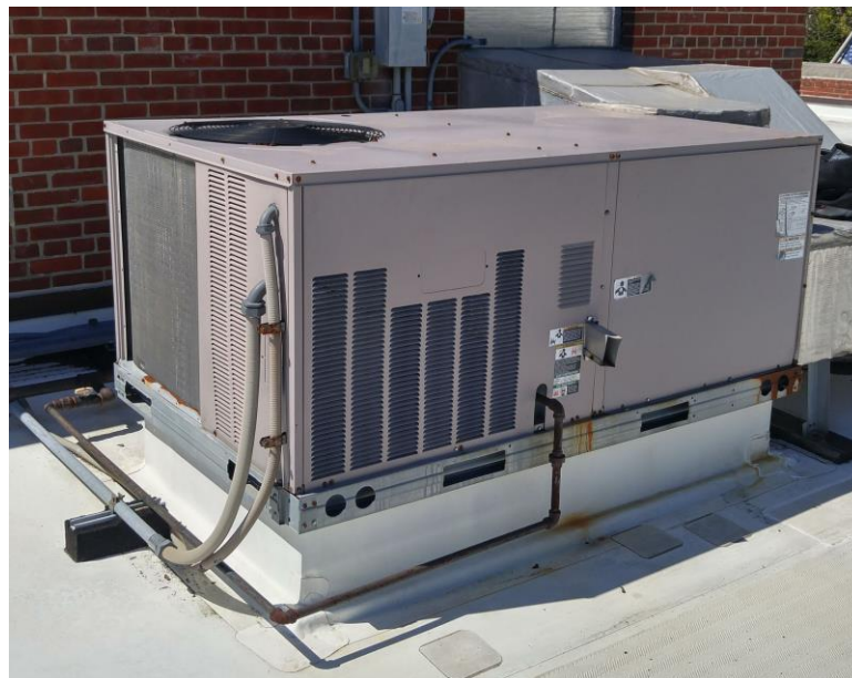
Photo 2 – Representative Rooftop Air Handler
