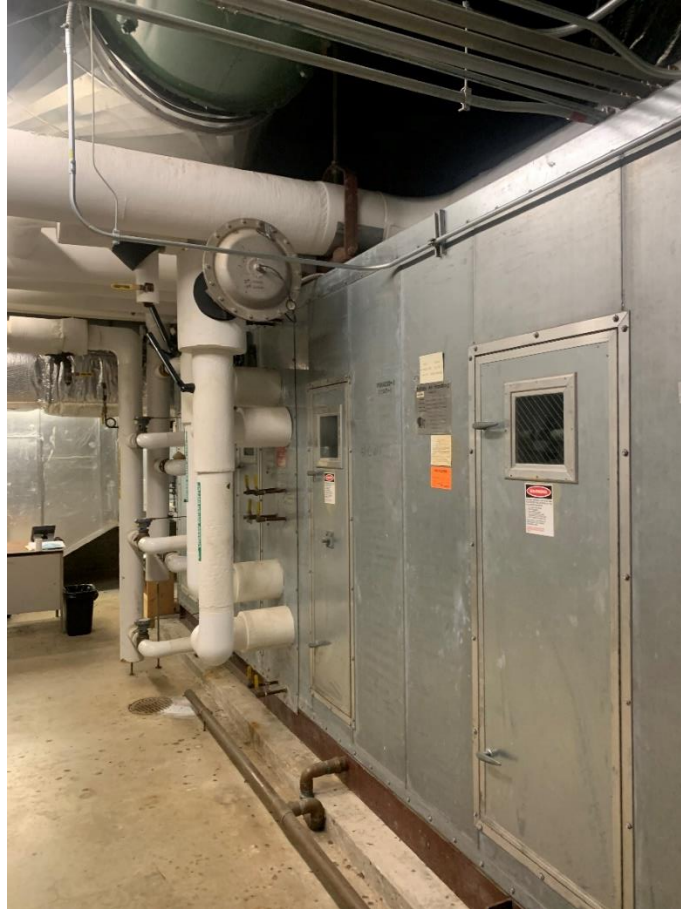
Photo 1 – Representative Air Handler
