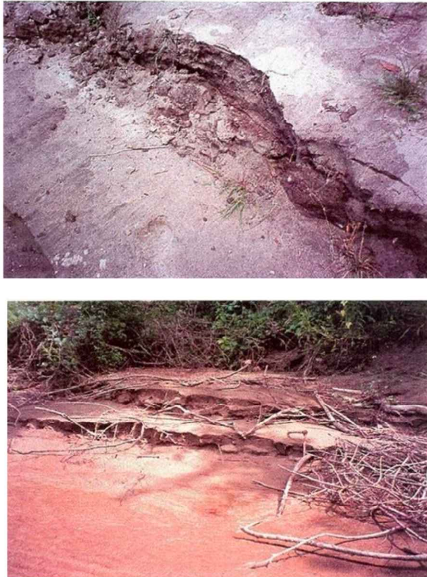
Figure 5.5.3-3: Notching Due to Boat Waves
