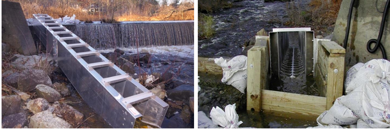
Alaska steppass fishway installed at Main Street Dam #4 on the Parker River in Byfield, MA (November, 2000)
