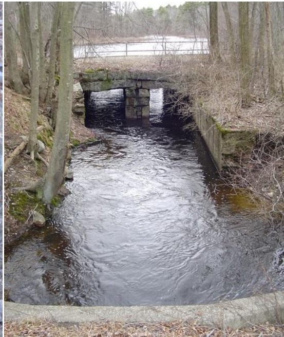
Looking upstream from Lake Street culvert to access road and culverts below Forge Pond Dam, with Forge Pond in background
