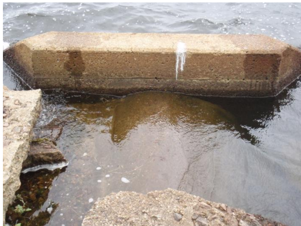
Monponsett Pond Diversion Pipe Outlet
