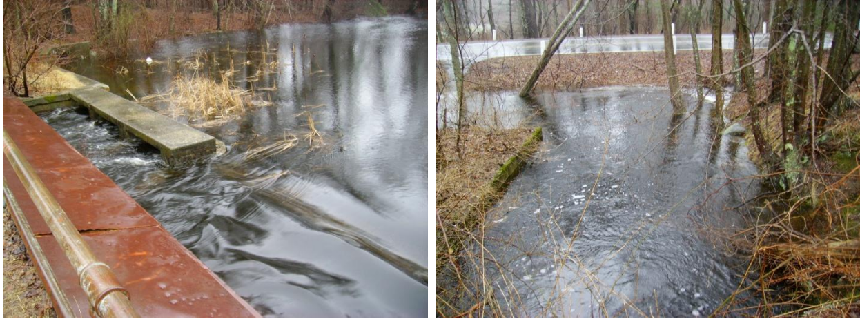
Photos taken during the March 15, 2010 flood at Forge Pond Dam from access road, looking upstream at submerged spillway (left) and downstream at submerged Lake Street culvert (right).
