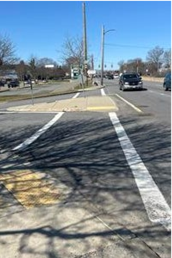
Missing Pedestrian Signal at the Route and Dean Road Intersection
