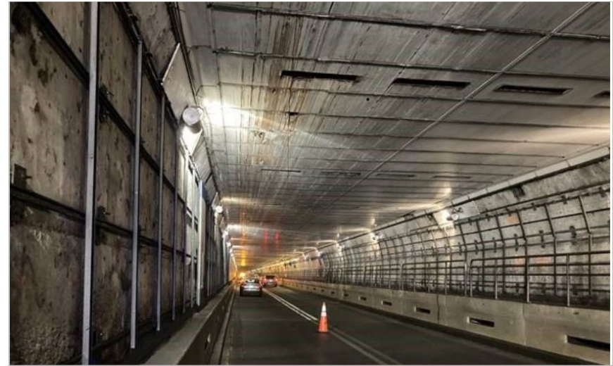
Sumner Tunnel before restoration
