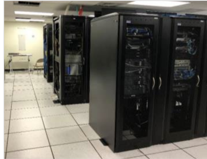
State Transportation Building server room
