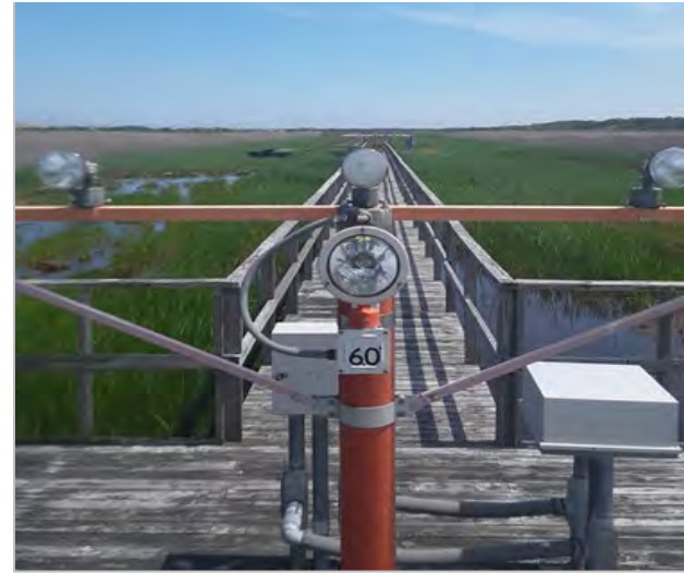
Provincetown Airport lighting
