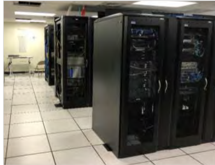
State Transportation Building server room
