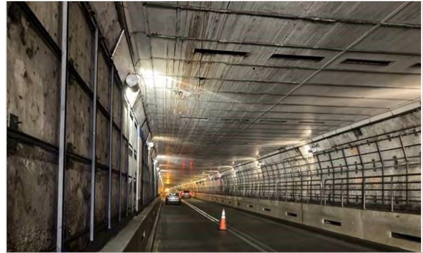
Sumner Tunnel before restoration
