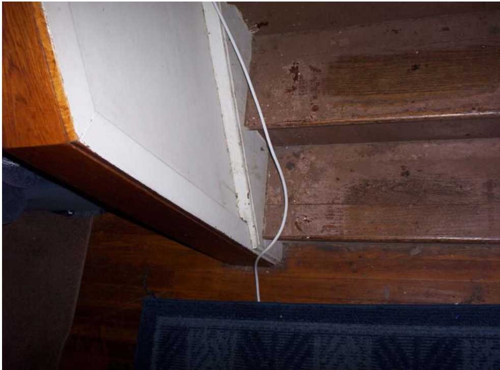
200-1 Development, 16 Patriots Circle Temporary Wiring on Stairs
