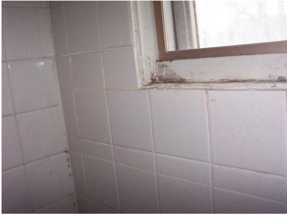
200-1 Development, 16 Patriots Circle Damaged Window Frame in Bathroom
