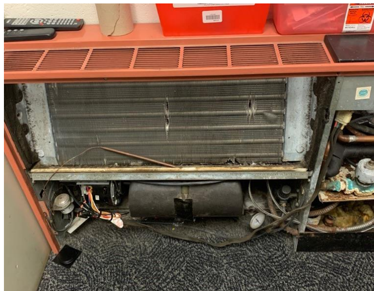
Photo 2 – Fan Coil with Cover Removed
