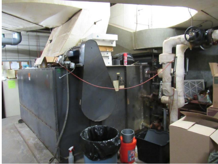
Photo 1 – AHU-1 Air Handler
