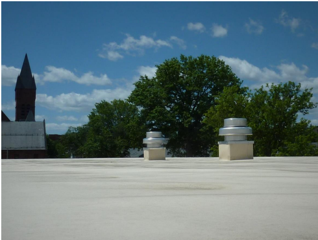
Photo 2 – Representative Exhaust Fans
