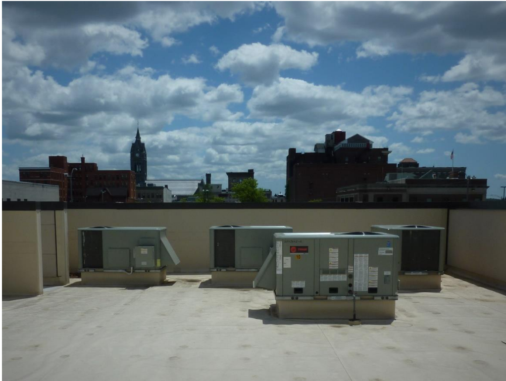
Photo 1 – Representative Rooftop Air Handlers
