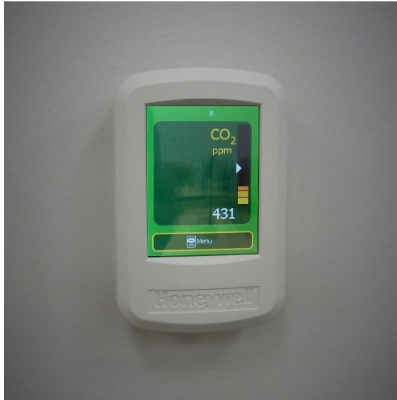
Photo 4 – Carbon Dioxide Sensor
