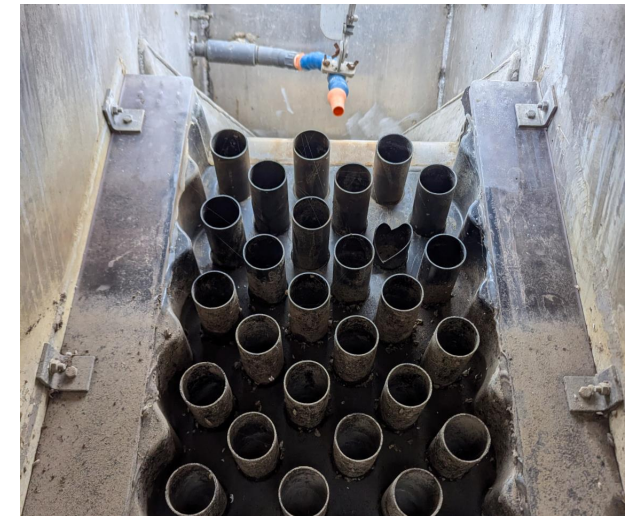
Eel Ladder, Saunders Dam, 2024
