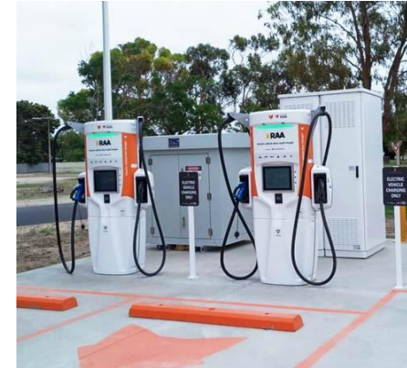
DC Fast Charging Stations (DC power)
