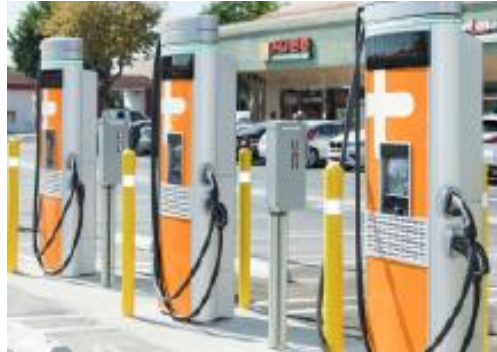
Level 2 Charging Stations (AC power)
