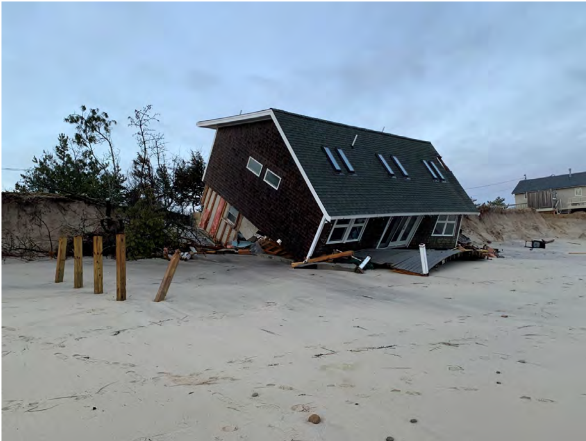
Photo courtesy of the Cape Cod Cooperative Extension/Woods Hole Sea Grant: solid wall foundation in V zone that collapsed from wave energy/erosion.
