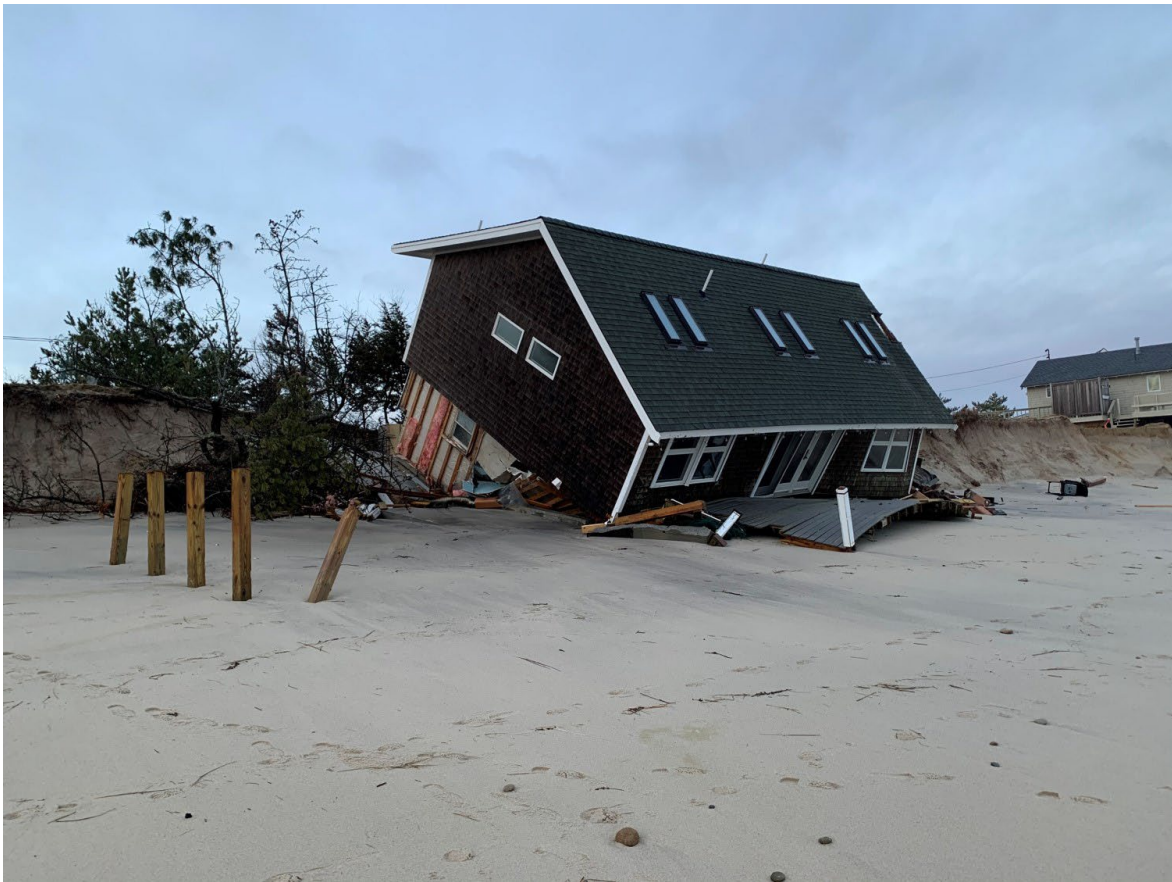
Figure 1: Photo courtesy of the Cape Cod Cooperative Extension/Woods Hole Sea Grant: solid wall foundation in V zone that collapsed from wave energy/erosion.
