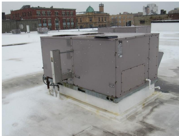
Photo 1 – Representative Rooftop Air Handler
