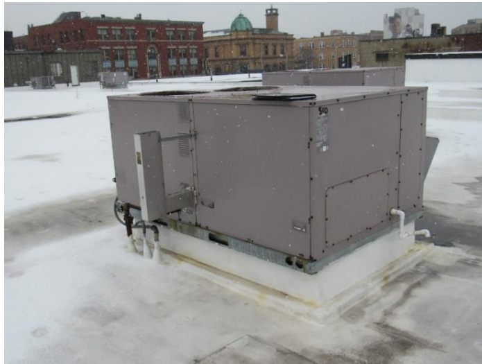
Photo 1 – Representative Rooftop Air Handler
