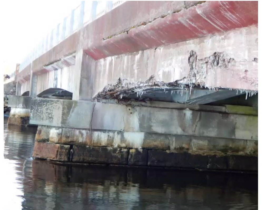
Existing conditions of deteriorating Marion-Wareham Bridge from underneath
