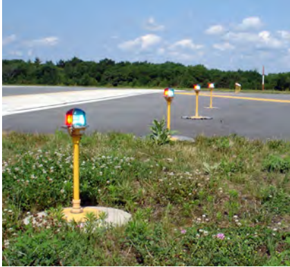
Runway end edge lighting
