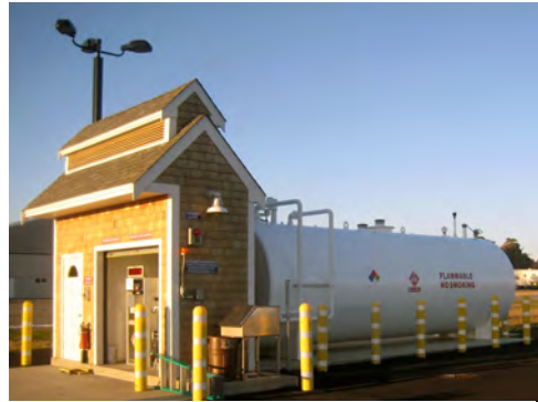
Fuel Farm (Chatham Municipal Airport)
