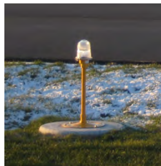
Runway Light (Chatham Municipal Airport)
