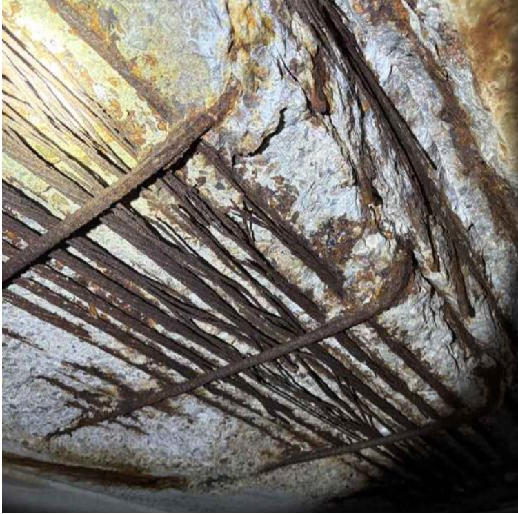
Figure 3: Severely Deteriorated Prestressed Concrete Butted Box Beams Showing Significant Loss of Concrete and Broken Prestressing Cables
