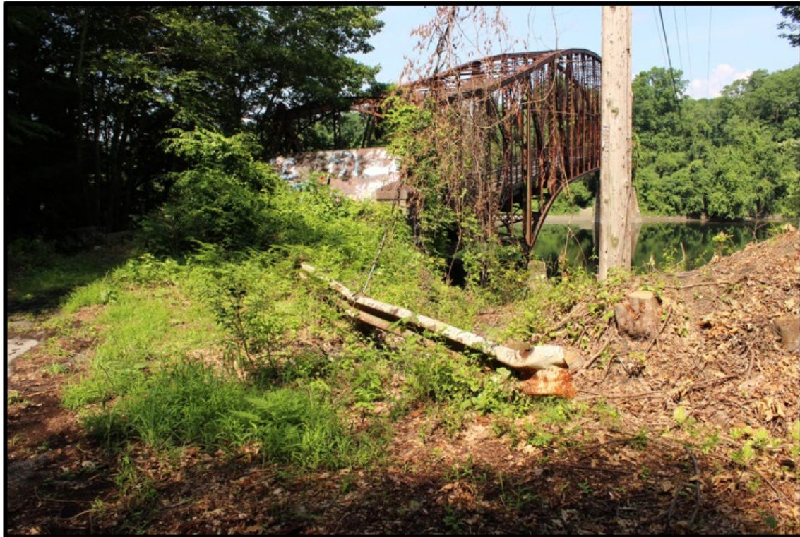
Existing Schell Bridge - Structurally Deficient Requires Full Replacement
