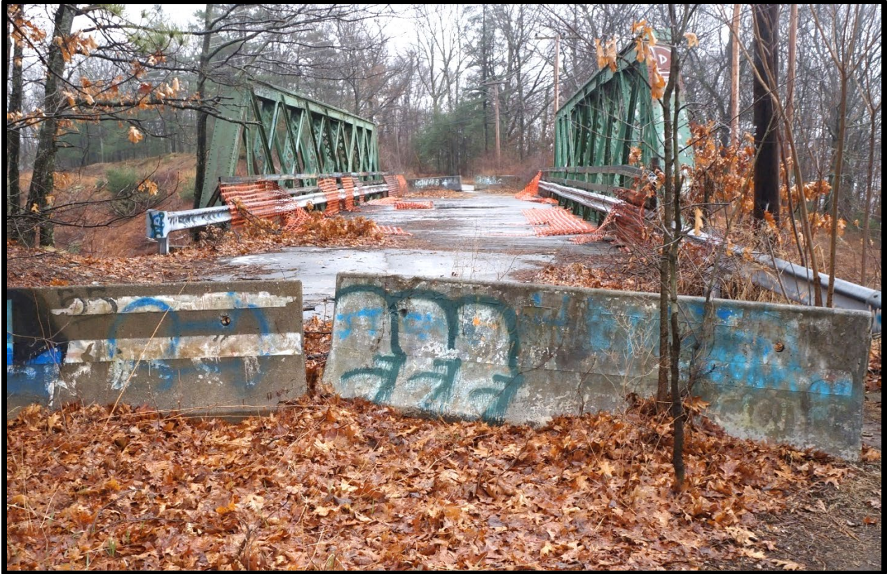
Existing Fisher Street Bridge - Structurally Deficient Requires Full Replacement
