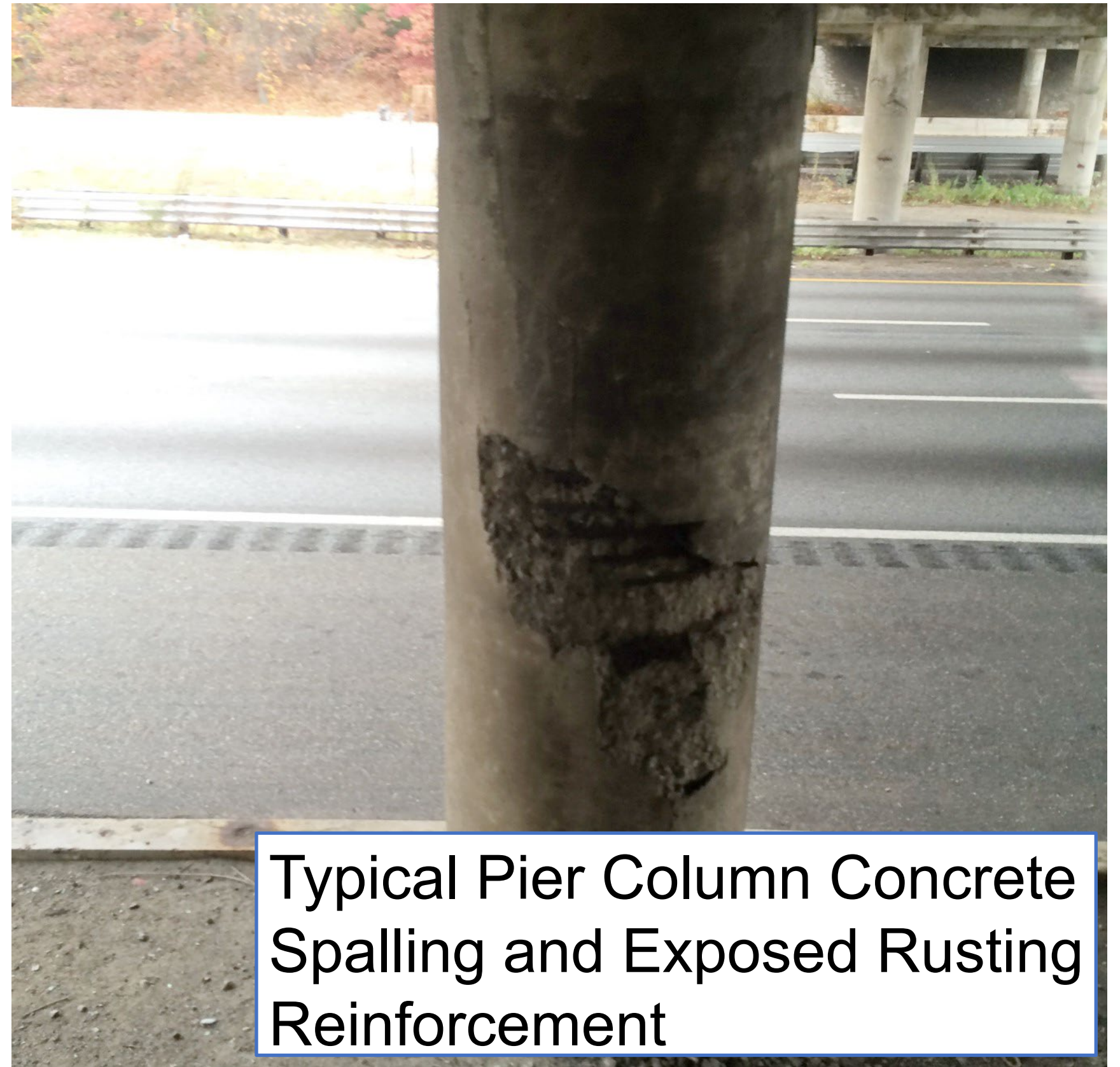
Typical Pier Cap Concrete Deterioration Showing Spalling and Cracking
