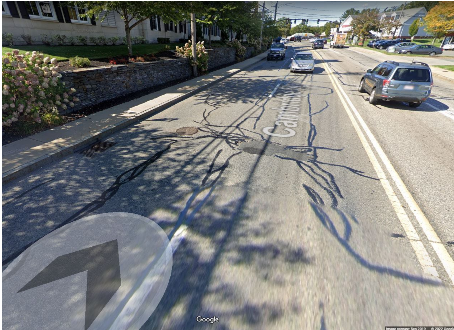
Screenshot from Google Maps showing typical pavement condition
