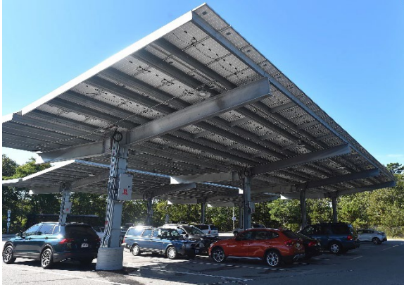
Solar panels at MassDOT Park & Ride
