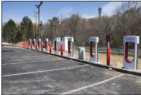
Charlton EV charging station
