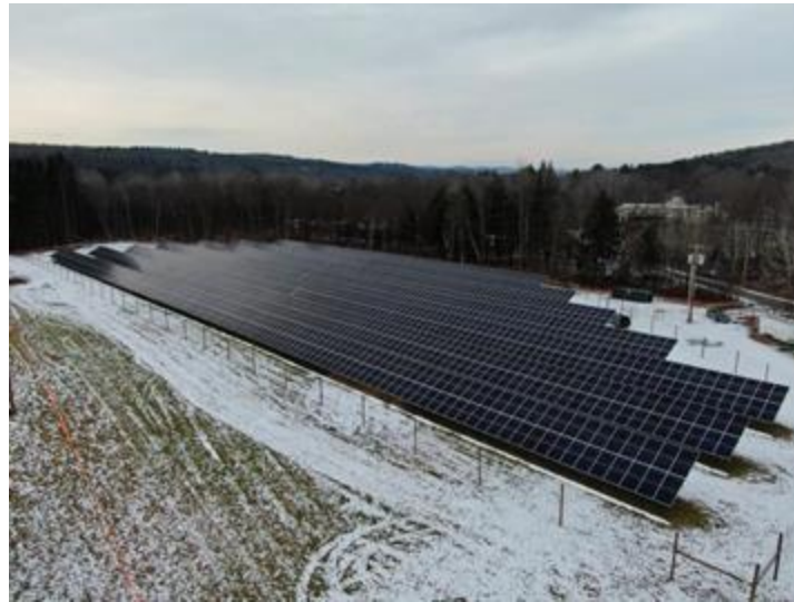
500 kW Class II Facility
