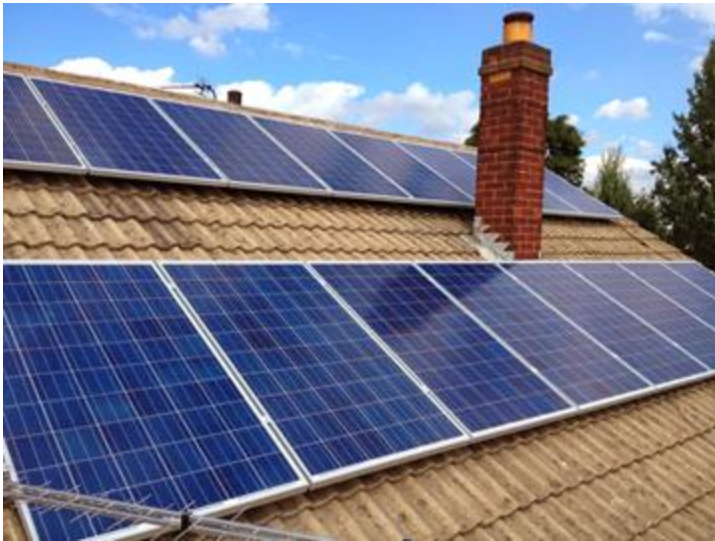
4 kW Class I Facility
